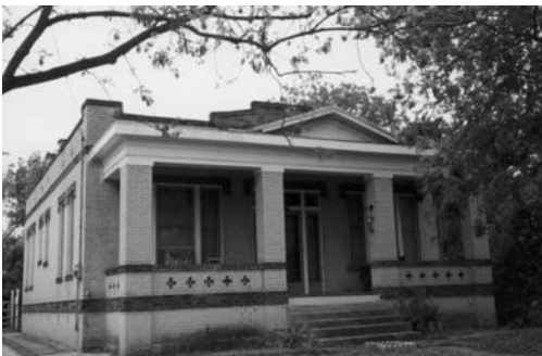
Brick wall surfaces should have deteriorated mortar replaced to keep moisture from entering the wall.
