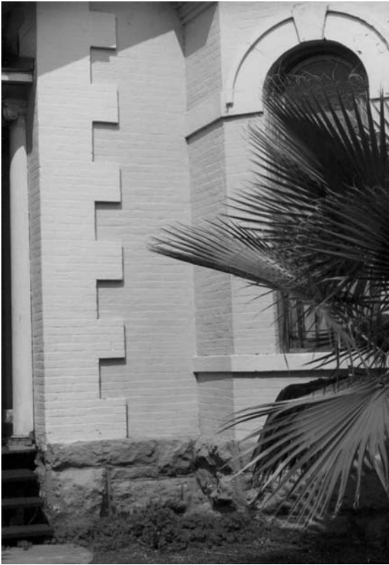
Stone perimeter beams or foundations last well over a hundred years if well maintained.
