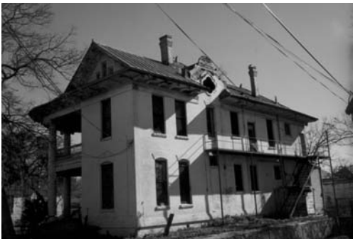
Painted brick surfaces can be cleaned and missing brick replaced to restore the wall.
