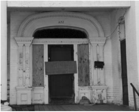
This detailed arched entrance with transom and side lights is important to the character of this house.
