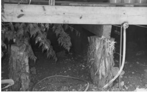
Pier and beam foundations are typical in Lavaca and are constructed with cedar posts and wood beams.
