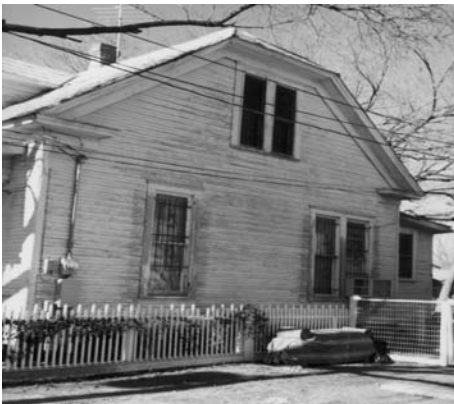
Deteriorated paint on wood siding should be properly removed during rehabilitation. The siding can then be primed and repainted for added life.
