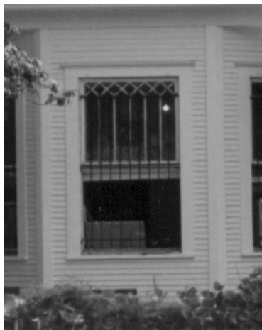
The multiple pieces of glass in a single sash are important to the character of this house.
