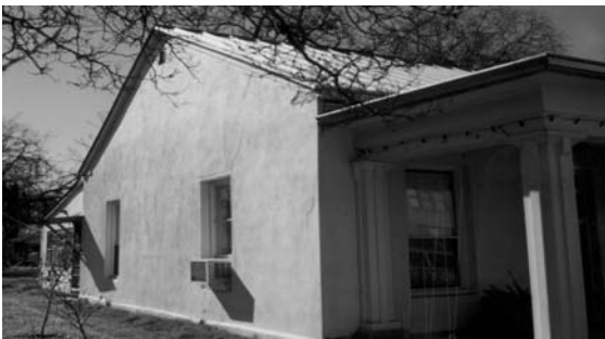
Portland cement plaster or stucco damages the stone underneath it.
