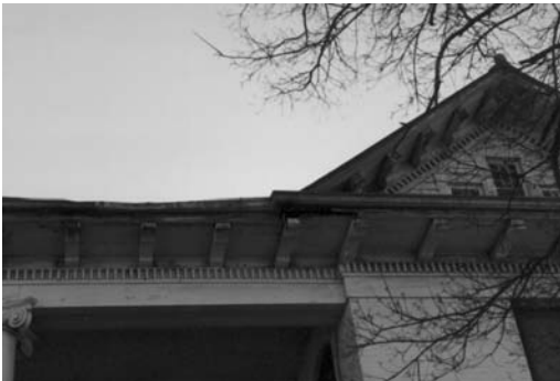
The deteriorated wood in the soffit should be replaced and the horizontal brackets reinstalled. Retain and repair the dentils and other detailing.
