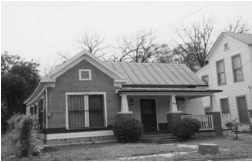
Existing synthetic siding could be removed and the wood siding beneath it could be restored.
