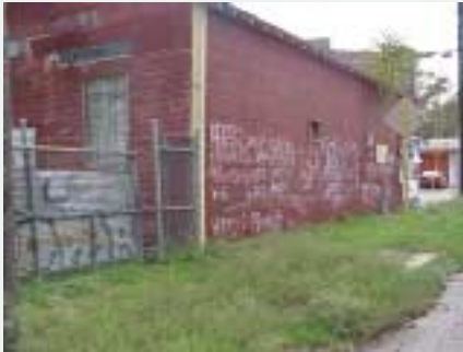
Example code compliance problem in the neighborhood
