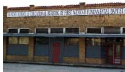
Non-conforming example of a commercial building that has window and door openings that have been partially covered with non-transparent materials
